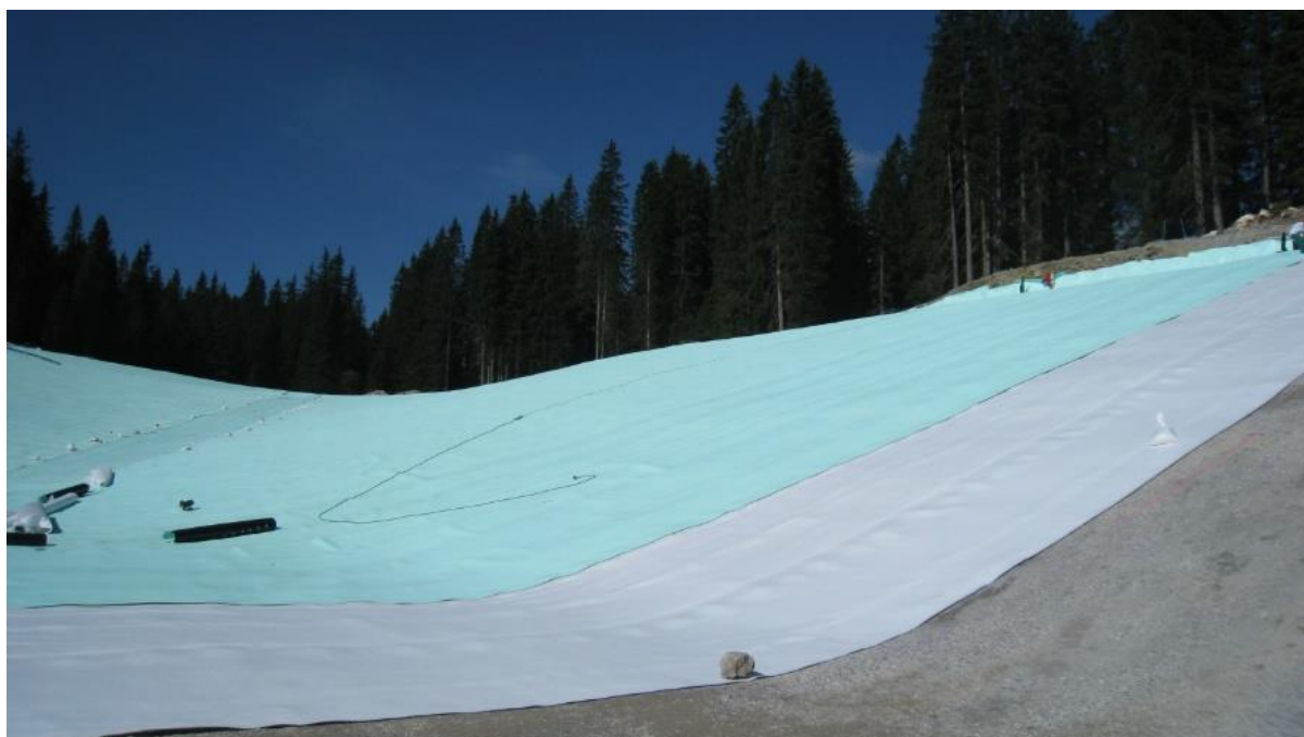
Figure 3:: Membrane MAPEPLAN T WT on water reservoir
